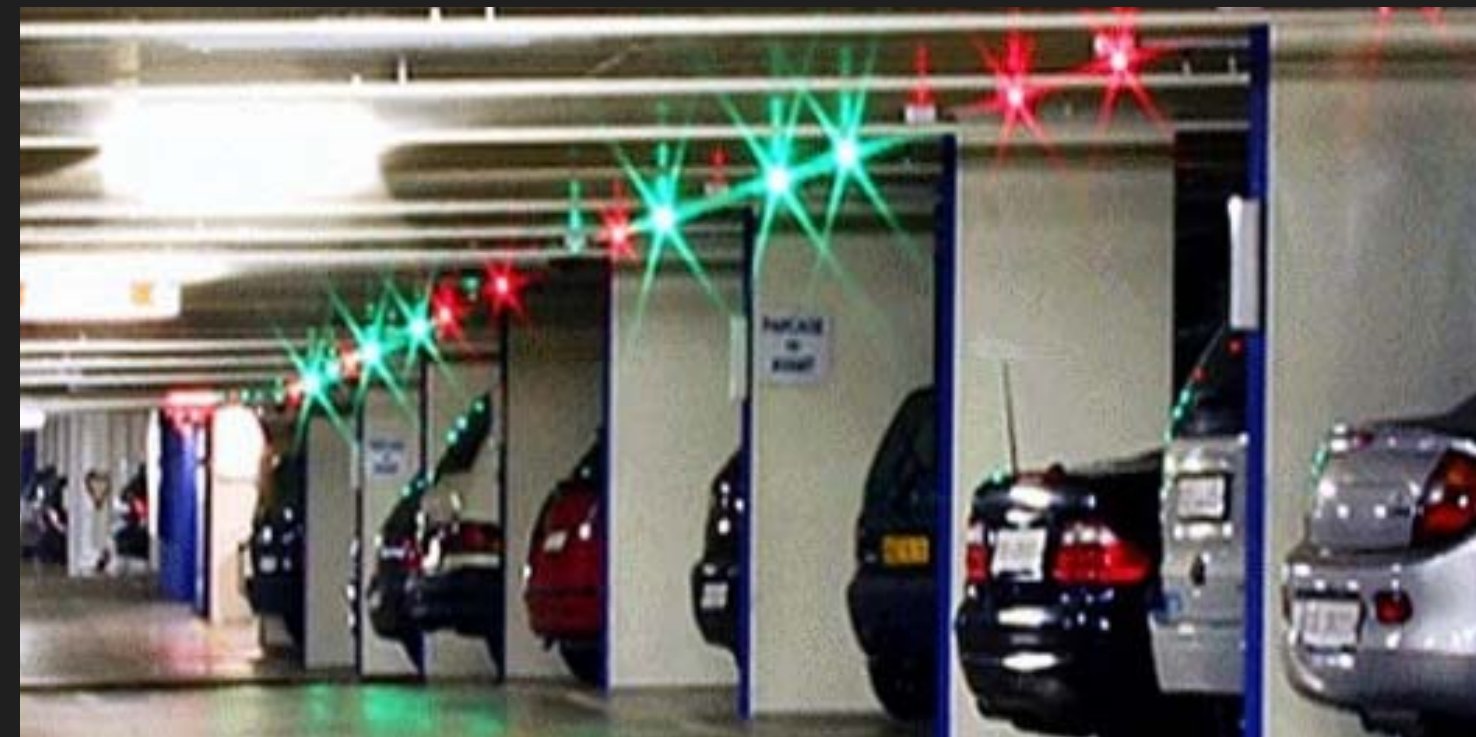
DEDICATED CAR PARKING MANAGEMENT SYSTEM FOR RETAILERS
