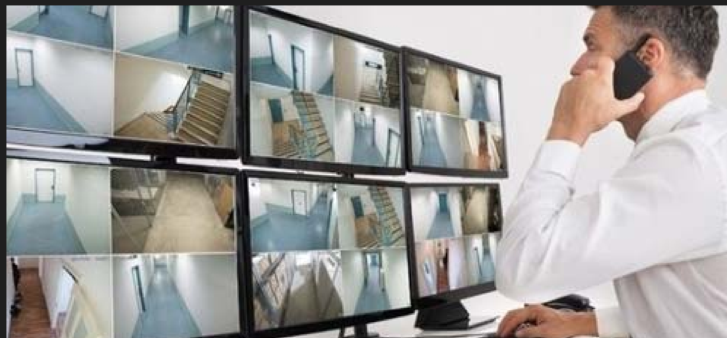
DEDICATED CCTV CONTROL ROOM
